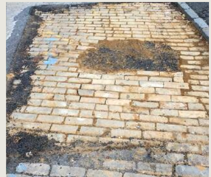
Damaged section of a yellow brick road.
